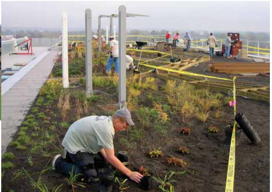
The green roof on the Clinton Presidential Library begins to take shape.
